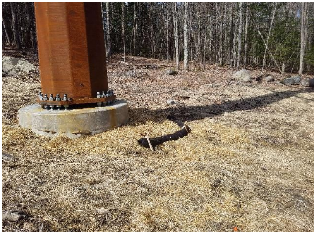
Fig 14: Erosion addressed at Str. 29, filter sock installed downslope of foundation. Viewing west. (03-31-20).
