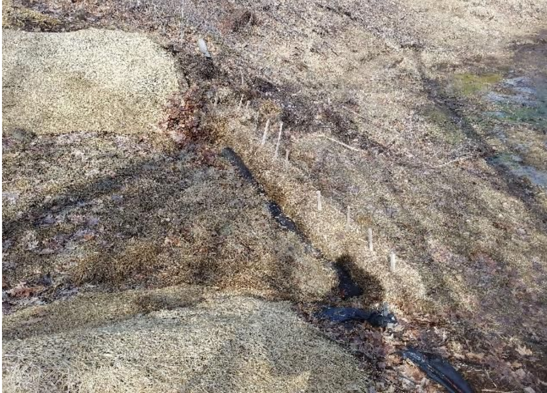
Fig 13: Filter sock installed on upslope side of bales on access road to Str. 28. Viewing east. (03-31-20).
