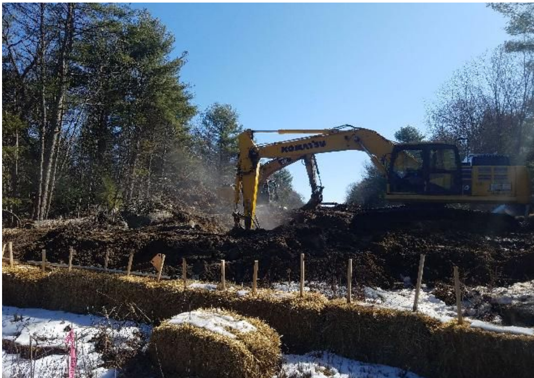
Fig 2: Hammering ledge at Str. 75. Viewing northeast. (03-26-20).
