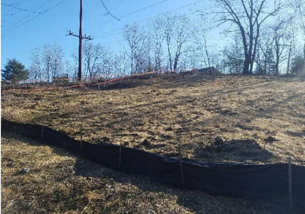
Fig 5: Soil pile blended into existing slope and area restored at Str. 27. Viewing northeast. (03-27-20).
