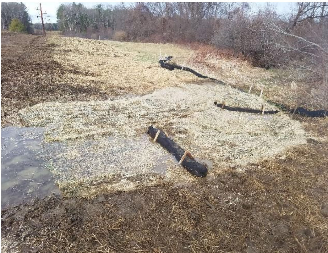
Fig 10: Repairs made to erosion in wetland NW18 at Frink farm. Viewing northwest. (03-31-20).
